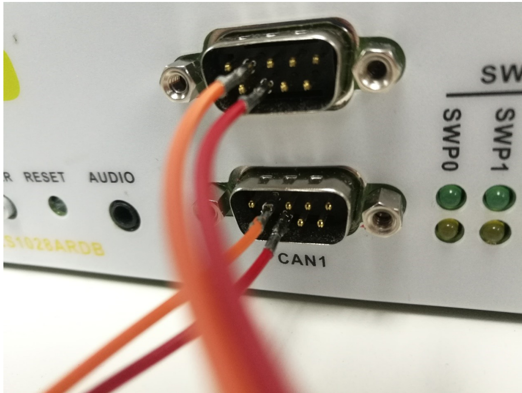
Figure 45. Physical connection for CAN using LS1028ARDB
