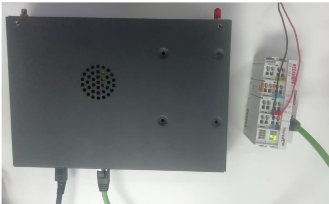
Figure 32. Board connects with BECKHOFF
